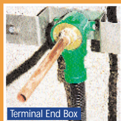
Terminal End Box
